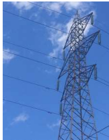
Fig. 4. 154 kV İkitelli-Yenibosna 1-2 Double Circuit Overhead Transmission Line RA1+15 Tower Photography
