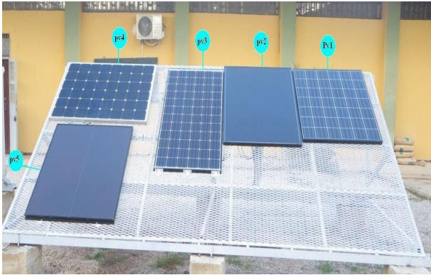
Figure 2 shows a photo of the 5 different technologies of PV modules installed in University of Saida (Algeria) and
